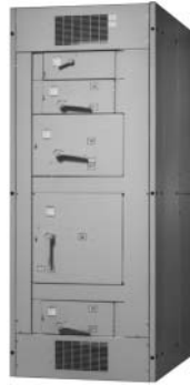
Front View—Fusible Units
